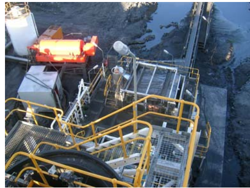
Belt Filter Area Prior to Rectification Works Project Development
