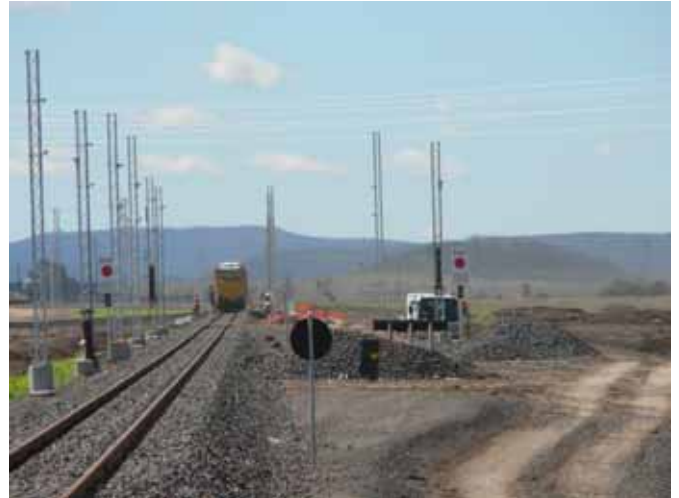
Overhead cabling to rail loop
